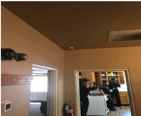
FIGURE 3-5: Battery Operated Smoke Detectors in most KCFD Fire Stations
