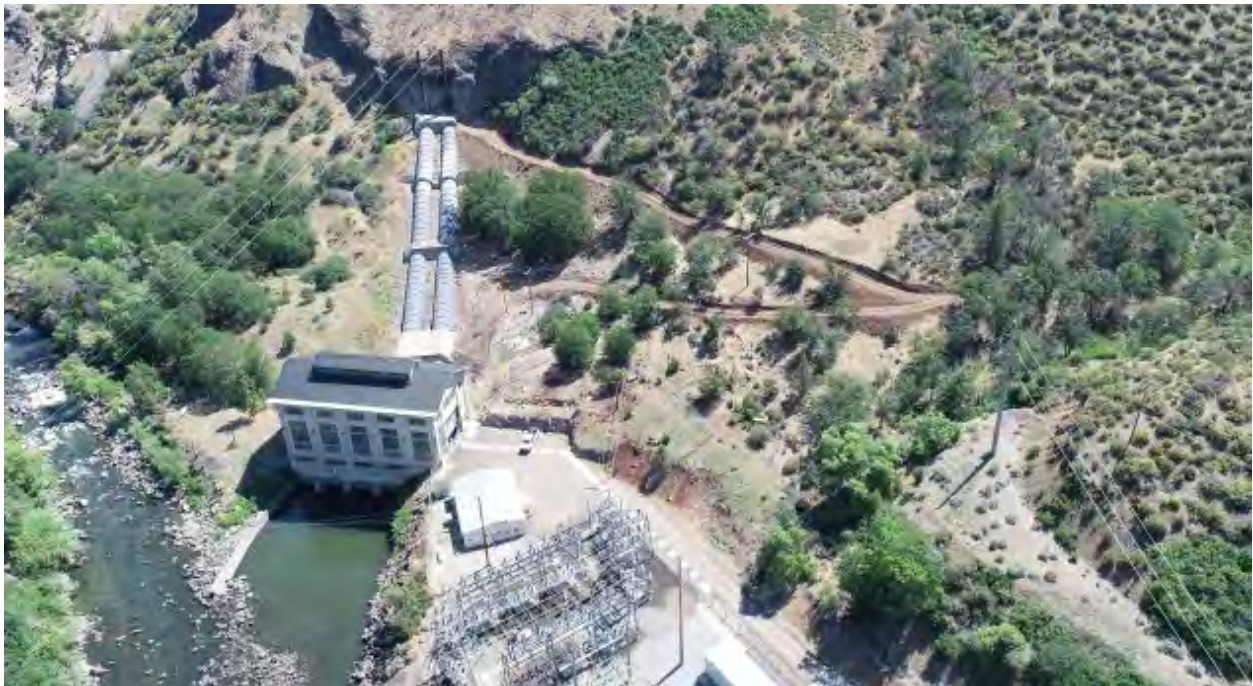
Access roads to the Copco No. 2 steel penstocks have been pioneered to facilitate demolition.
