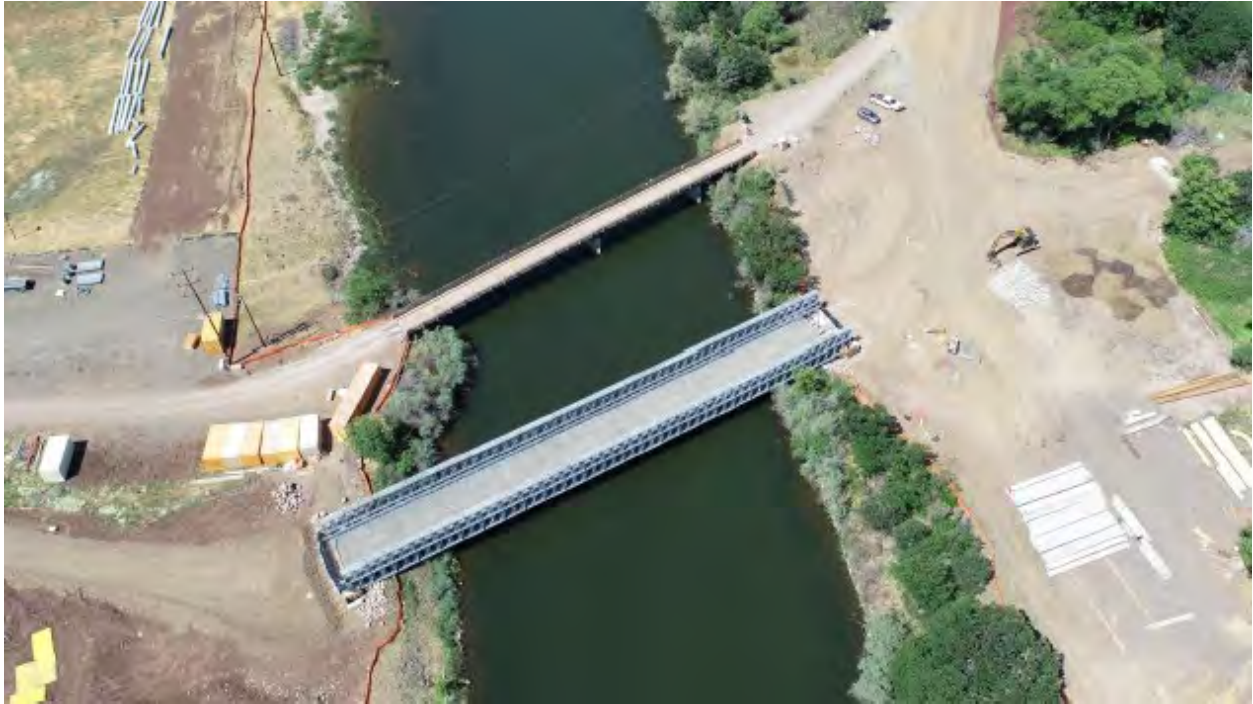
Daggett Bridge after installing the decking. Remaining abutment walls have been poured at each end.
