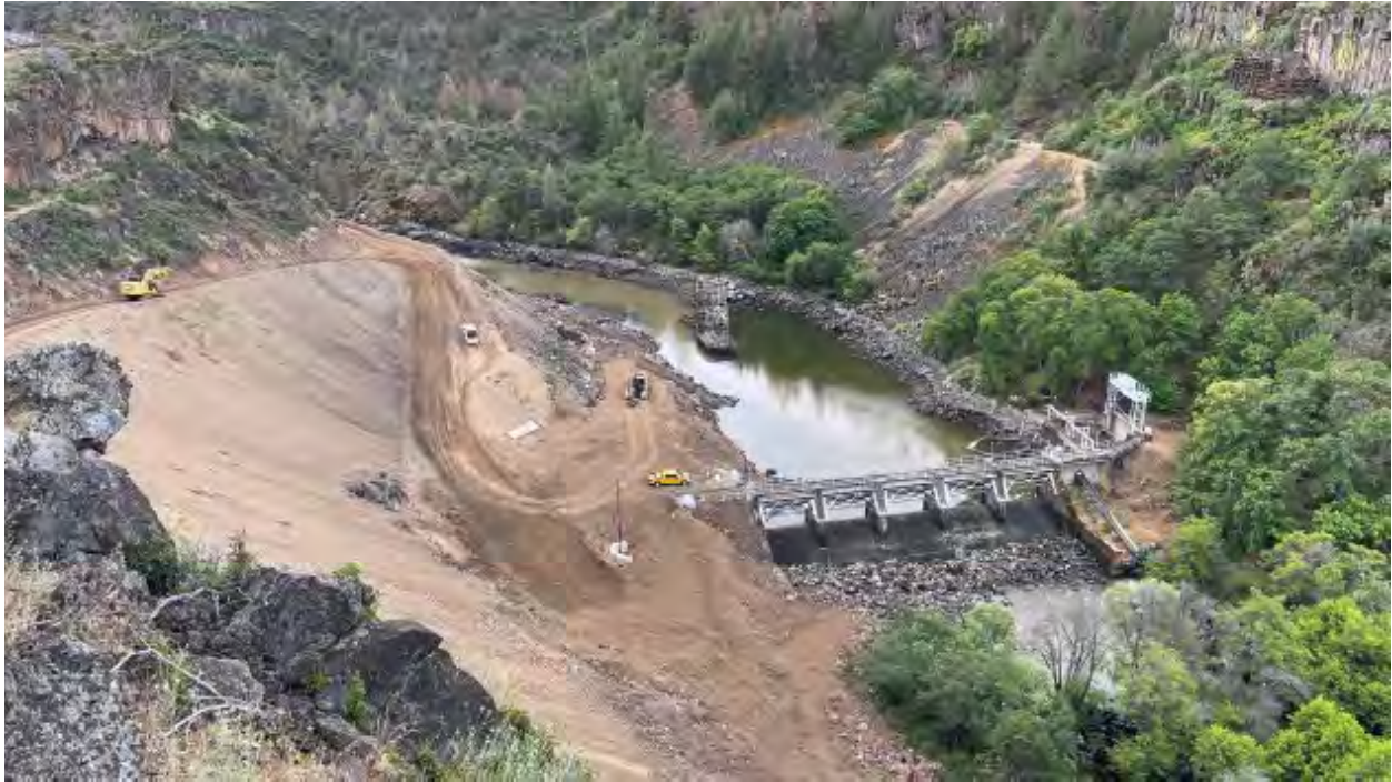
Copco No. 2 dam (foreground) and historic wooden diversion structure (background) after facility termination and handover but before demolition began.
