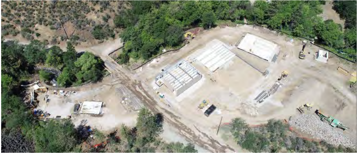
Fall Creek Hatchery progress. Placed concrete for Chinook raceways banks #5 through #8. Began erecting Chinook Incubation PEMB. Fish Ladder and Fish Barrier concrete placed.
