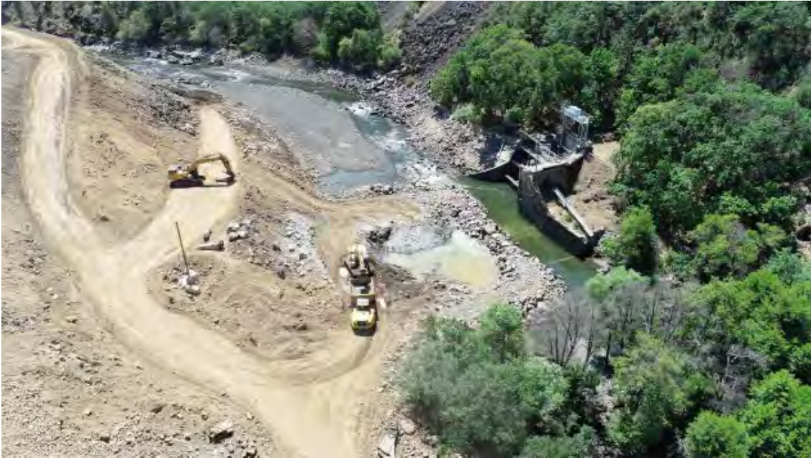
Aerial view showing progress on Copco No. 2 demolition at the end of June. The dam has been removed down to the foundation and removal will continue through the month of July. Note that the historic wooden diversion structure is completely removed in the background.
