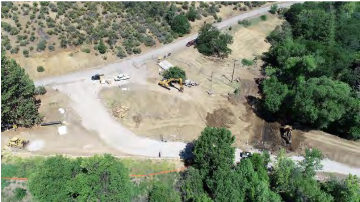
Construction started on the Fall Creek Culvert replacement. Shoefly road was constructed to route traffic around the work area.
