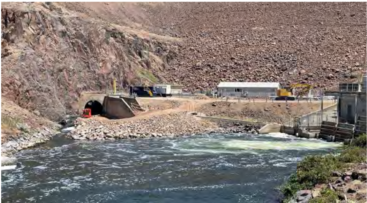
Access pad to the tunnel face at Iron Gate Dam has been constructed.
