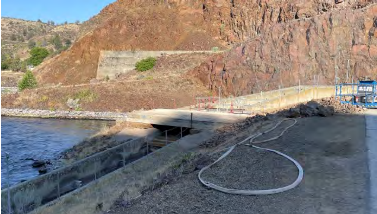
Initial construction of the temporary bridge over the fish ladder at Iron Gate Dam.
