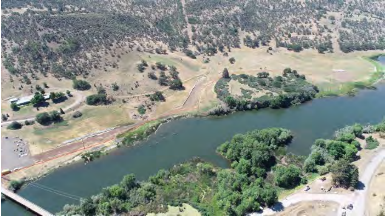
City of Yreka Waterline alignment has been cleared and grubbed and pipe laid out.
