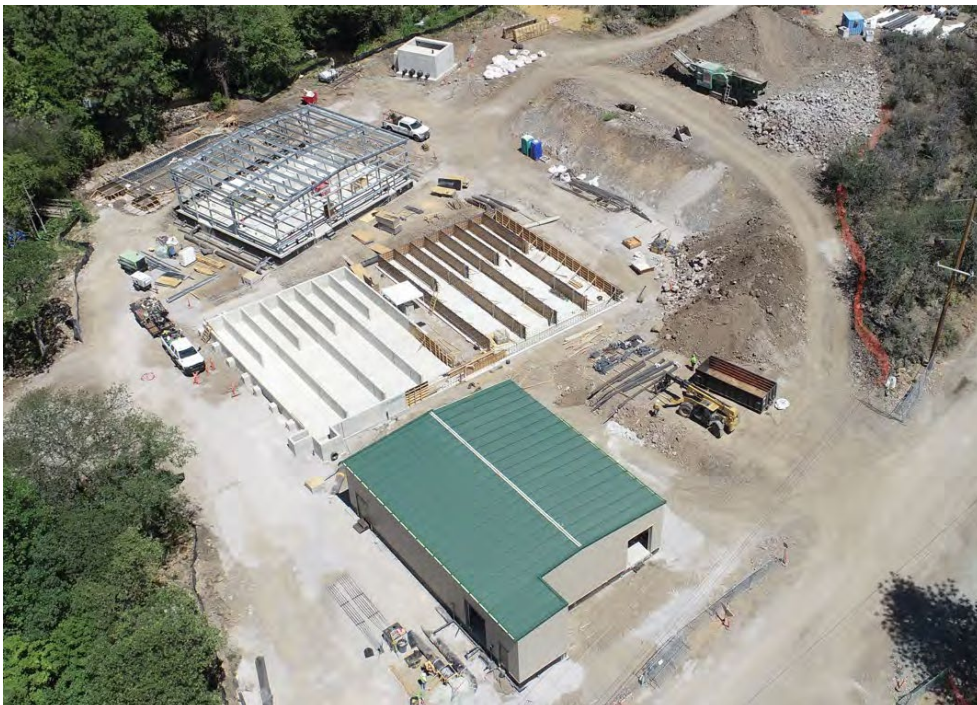
Fall Creek Hatchery progress. Chinook raceways banks #5 through #8 complete. Chinook Raceways #1 through #4 wall forms in place.
