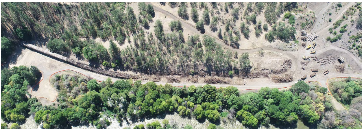
Aerial view showing Copco No. 2 wood stave flow line demolition. Wood staves are piled within the flowline alignment to contain contaminated materials.
