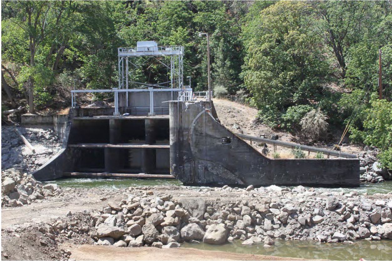
Aerial view showing Copco No. 2 demolition progress at the end of July. The dam and right abutment have been removed down to the foundation slab. The remaining demolition of the left abutment and foundation for final channel grading will be completed during weekly outages in September.
