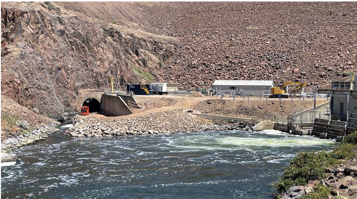
Access pad to the tunnel face has been constructed at Iron Gate Dam.
