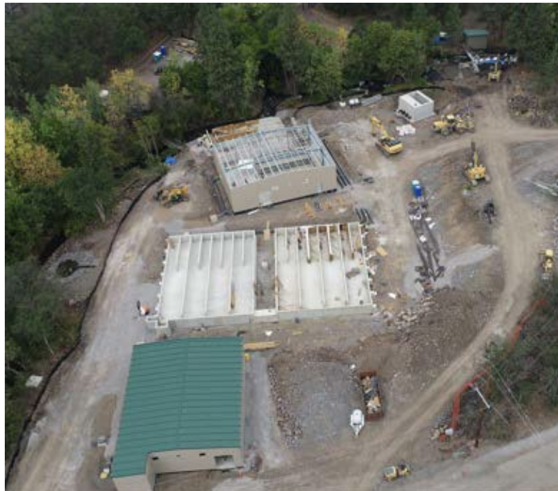
Fall Creek Hatchery progress. Chinook raceways banks #5 through #8 complete. Chinook Raceways #1 through #4 wall forms completed. Began erecting Coho Building PEMB. Began Adult Holding Pond formwork and rebar.
