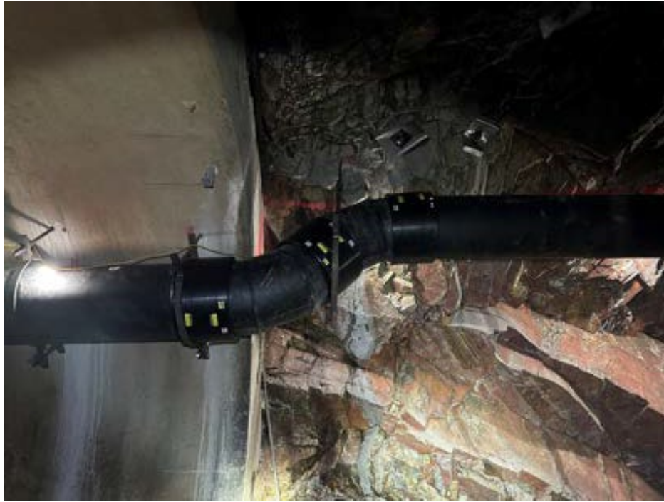
New HDPE vent line transition from lined to unlined tunnel at Iron Gate.
