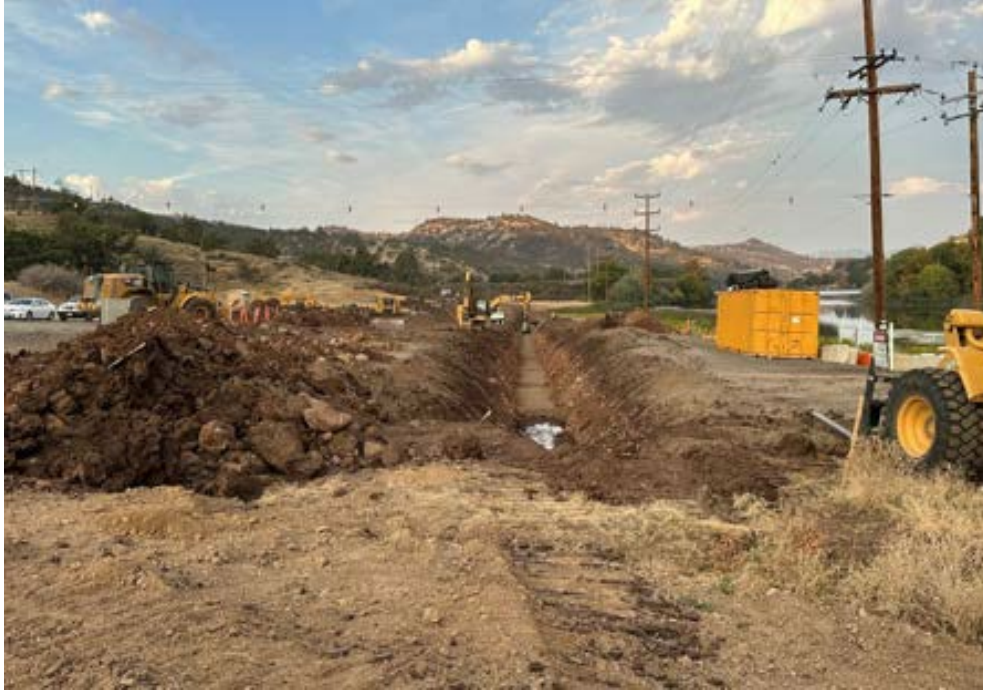
City of Yreka Waterline crossing Daggett Road.
