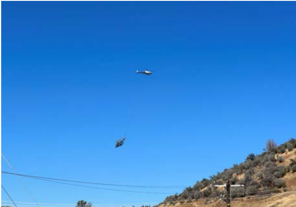
Helicopter flying trees from Ward's Canyon to the staging and storage area.
