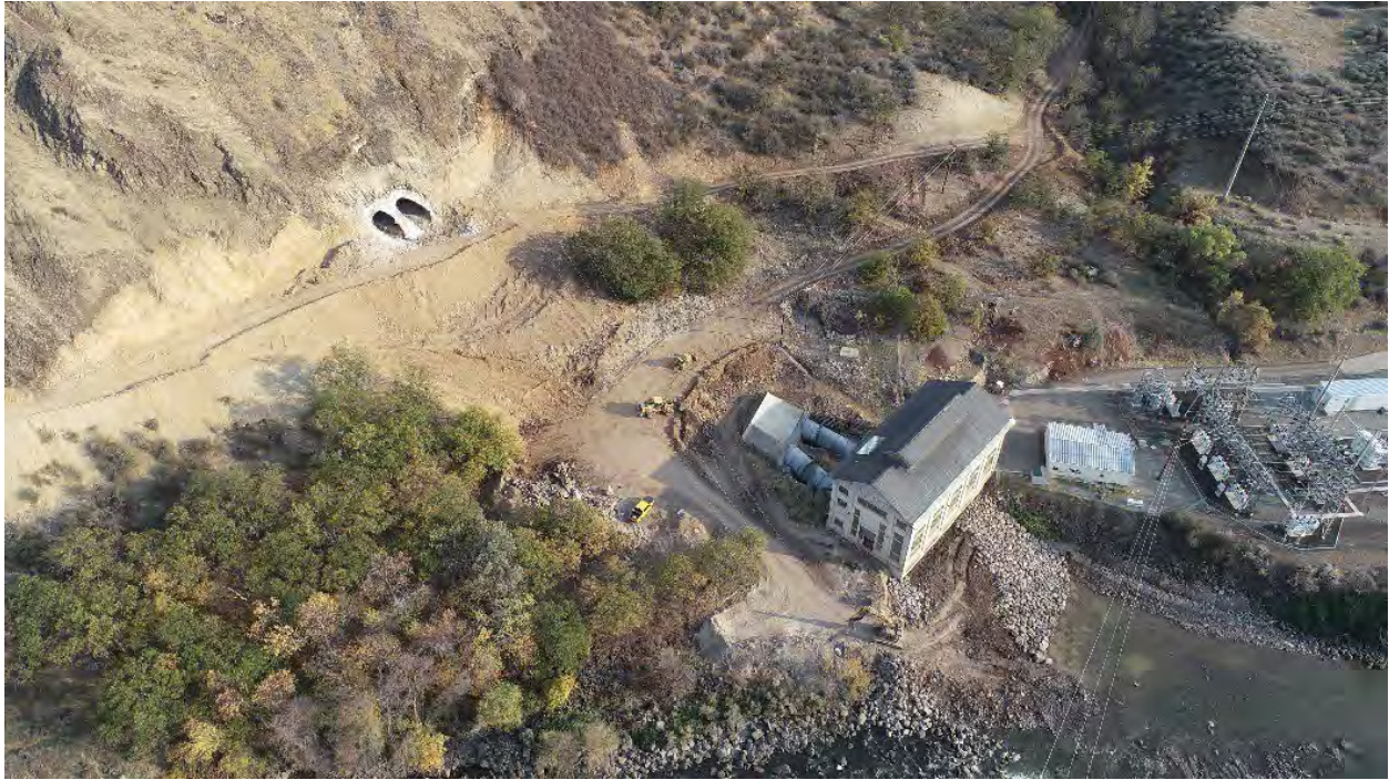
Copco 2 steel penstock thrust blocks have been removed. Lower thrust block backfilled. Tailrace filled and rip rap being placed.
