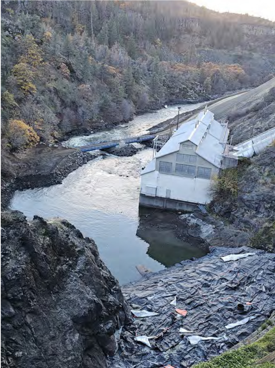
General view of Copco 1 dam and powerhouse with bridge access to diversion tunnel outlet and completed grouted riprap pad over steel extension pipe.
