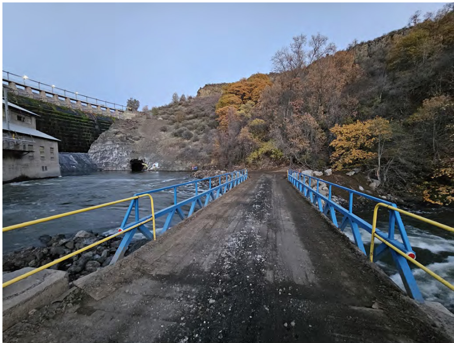
General view of Copco 1 dam and powerhouse Jim Bob bridge access to the diversion tunnel outlet.
