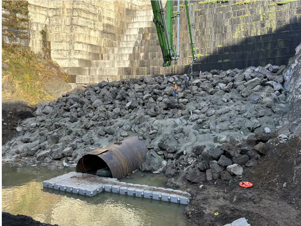
Stell extension pipe at Copco 1.
