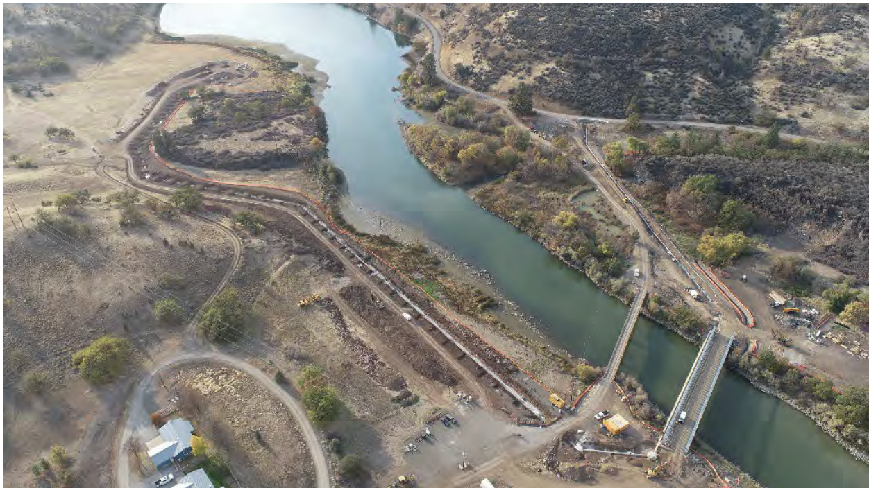
Aerial view of City of Yreka Waterline progress. Excavation and pipe laying are complete.
