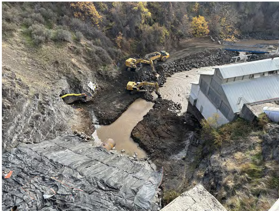
General view of Copco 1 dam and powerhouse with progress removal of access pad to steel extension pipe and low-level adit.
