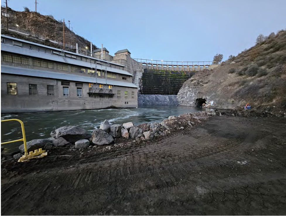
General view of Copco 1 dam and powerhouse with access pad to steel extension pipe and low-level adit removed.
