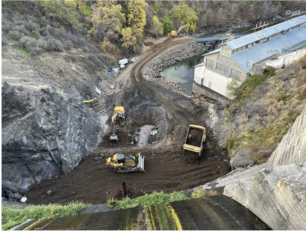
General view of Copco 1 Dam and Powerhouse with progress on fill over steel pipe extension.
