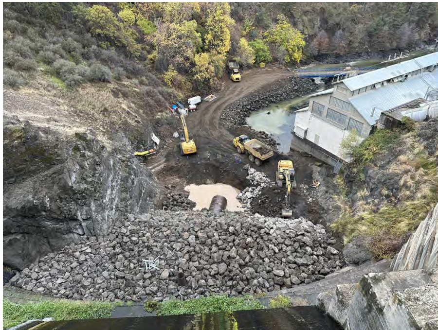
General view of Copco 1 Dam and Powerhouse with progress on riprap placement over steel pipe extension.
