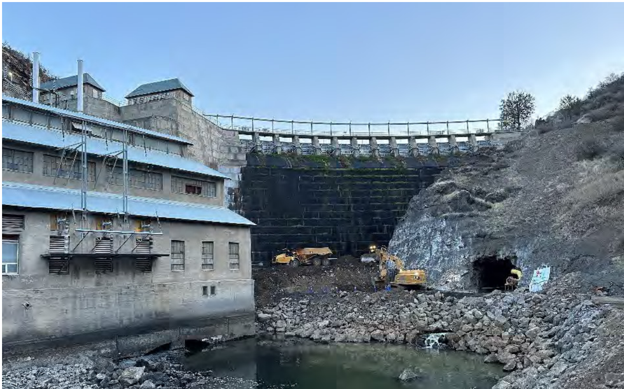
General view of Copco 1 Dam and Powerhouse with progress on fill over the steel extension pipe.
