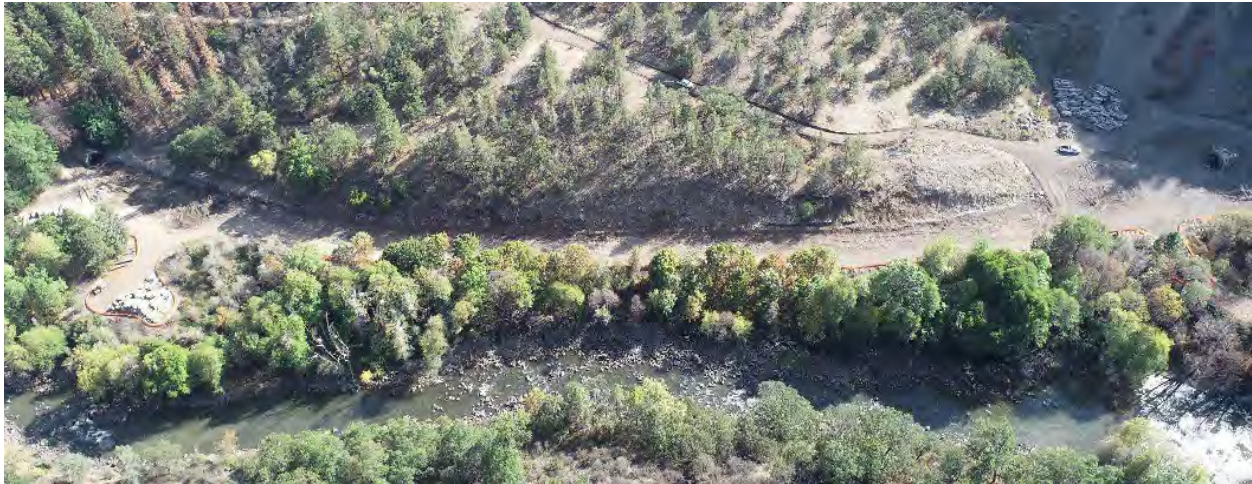
Copco 2 wood stave flowline demolition complete. Concrete supports have been removed and placed to the side in preparation for soil remediation contractor.
