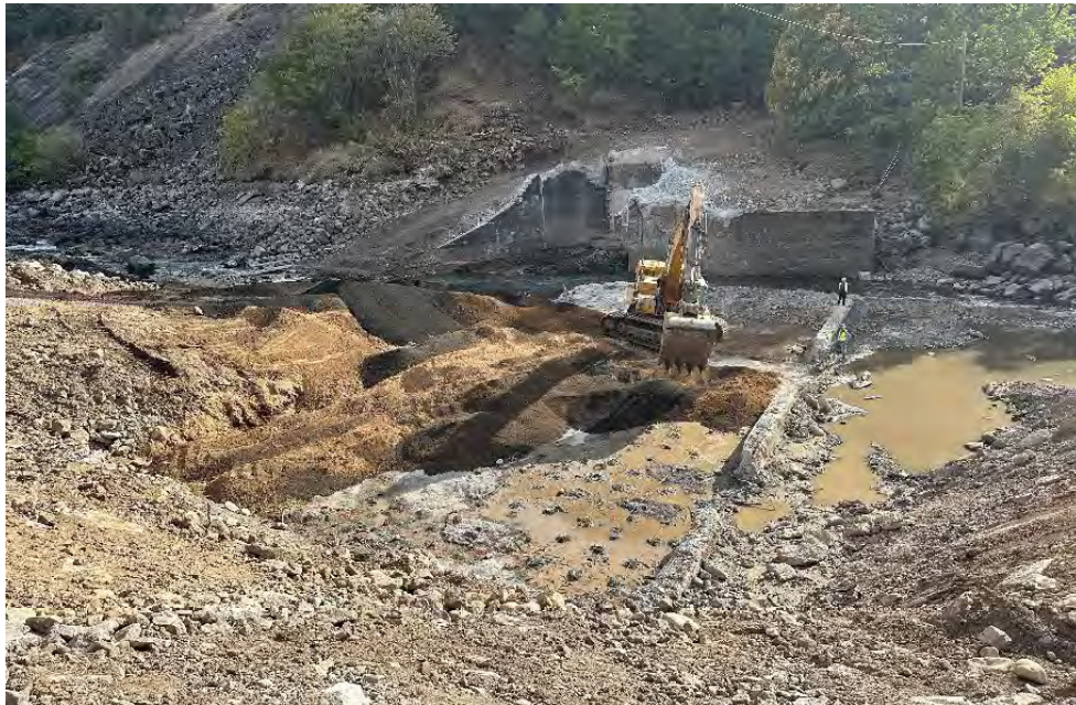
Covering loaded holes with earth fill before first blast at Copco 2 foundation.
