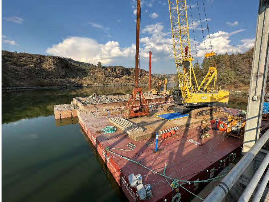
Dredging and debris barges moored at Copco 1 Dam while dredging in front of the new low-level adit. Debris, including rock and timbers can be seen in the debris barge.
