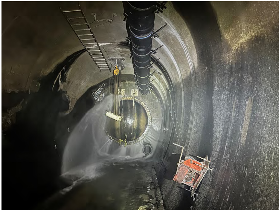
Blind flange closed and new HDPE vent line installed in the tunnel ceiling of Iron Gate.
