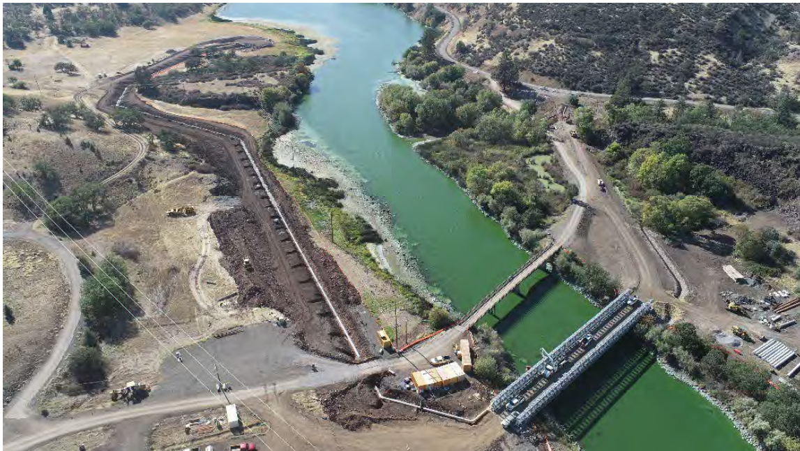
Aerial view of City of Yreka Waterline progress. Excavation is completed from the downstream tie-in to the new Daggett Bridge, and excavation is starting near the upstream tie-in. Pipe has been laid and welded from the downstream tie-in to the new Daggett Bridge and is currently being laid across the bridge.
