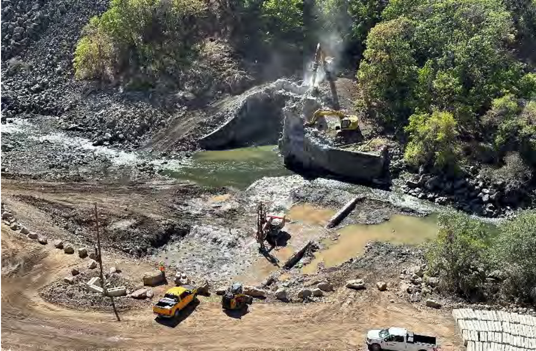
Background: demolition of the Copco 2 dam intake structure and left abutment. Foreground: drilling holes in preparation for blasting Copco 2 dam and spillway foundation.
