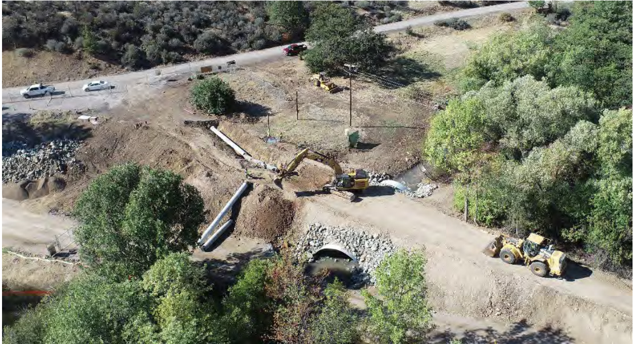
Beginning to excavate and lay pipe near the upstream tie-in and the Fall Creek Culvert.
