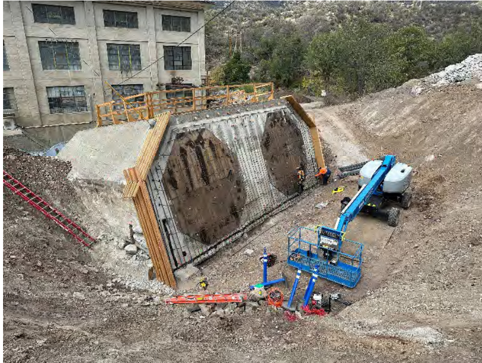
Copco 2 lower thrust block framework and rebar installation for permanent concrete plug.
